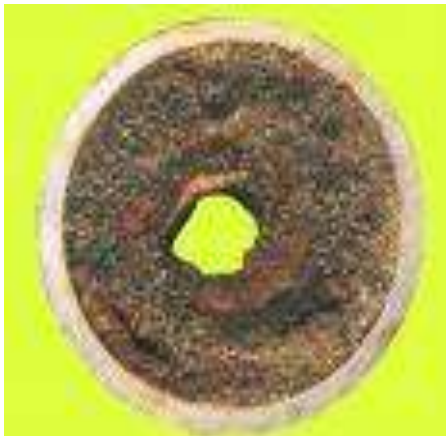
Section of a pipeline with deposited wax
